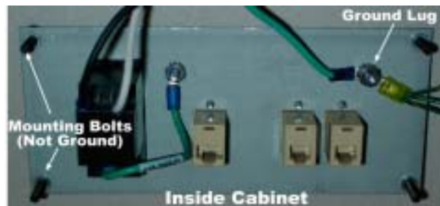
Figure 2. Cabinet Power Plate
