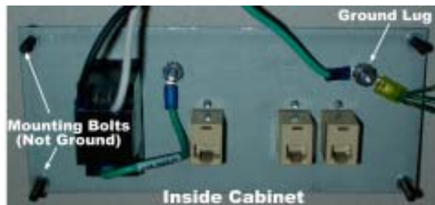
Figure 2. Cabinet Power Plate
