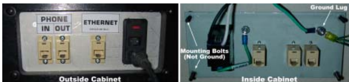
Figure 44. AC Power Plate (Standard Cabinet)
