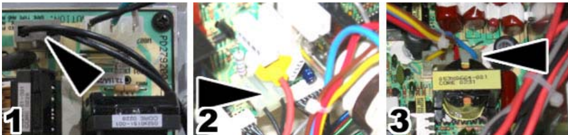
Figure 11. Monitor PCB Cables
