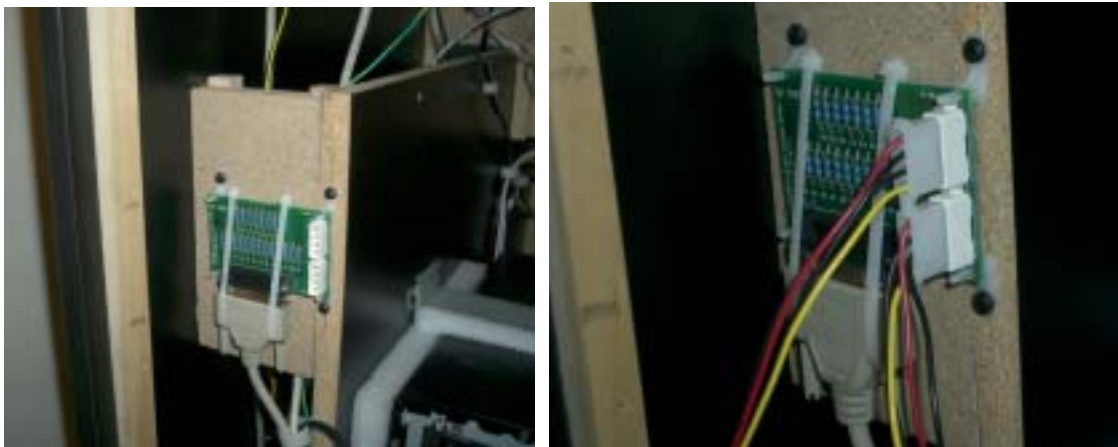
Figure 3. Header Controller Board Installation
