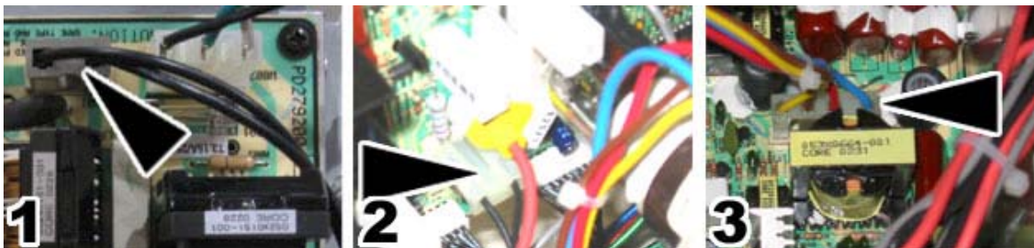
Figure 23. Monitor PCB Cables
